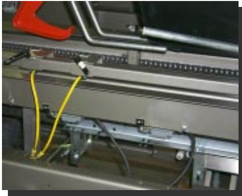
figure 20-3. Gate Enable and F.B. Disable Switches and Kicker Photoeyes
