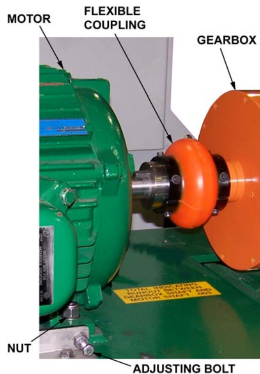
Figure 5-3 Conveyor Drive Flex Coupling
