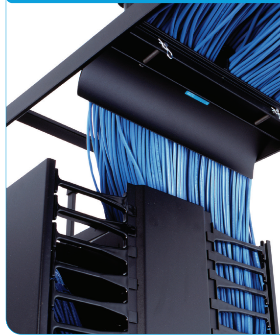
Cable Management Bend Radius Category 6A cables
